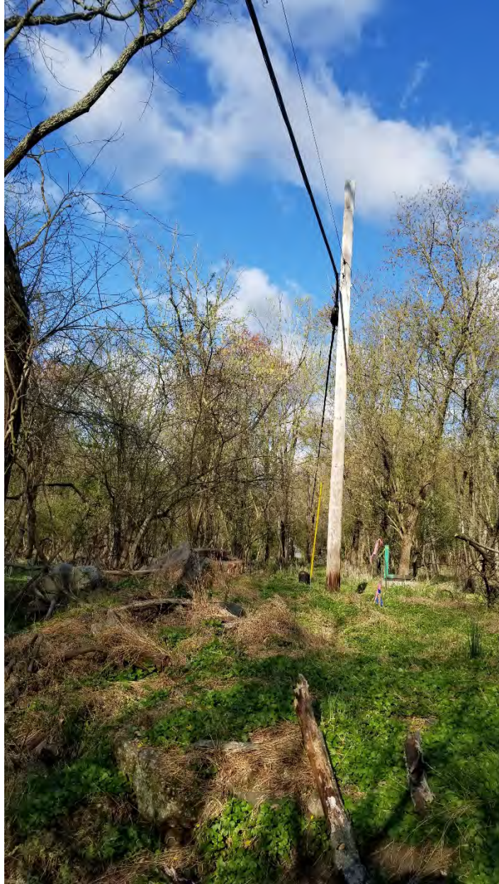
Photo 5: Electric lines running over the unnamed tributary.
