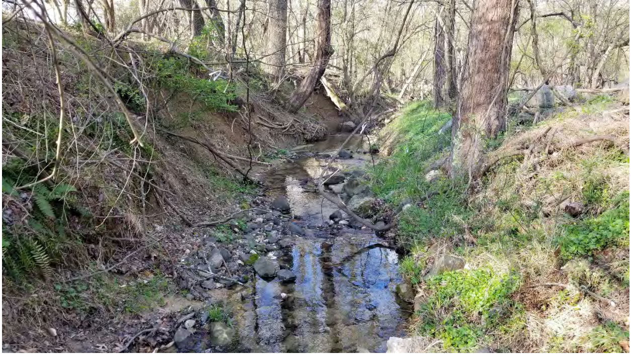
Photo 3: The left bank of the unnamed tributary is near vertical and lacking vegetation with a rooting depth that would assist in bank stabilization. The bank is approximately 4 feet tall.
